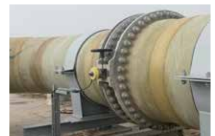
Gas ventilation and scrubber
