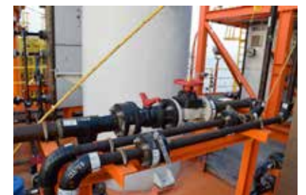
FPSO (Sodium hypochlorite processing)
